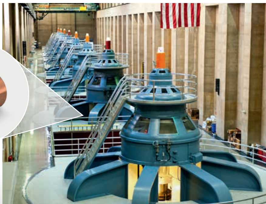
Turbine Hoover Damm
