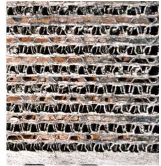
Clogged cooler fins
